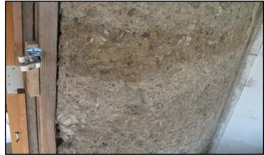
House wall made of clay, sand, straw, and manure at Sunbow Farms.
